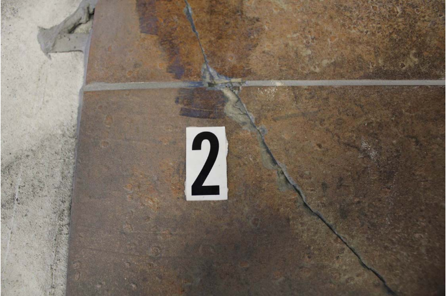
Image 4: Broken tile and spalled grout joint
